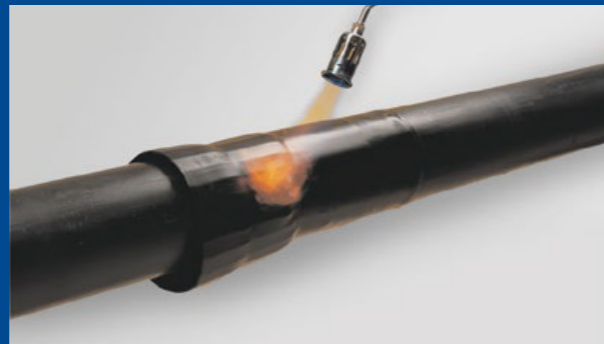
Shrinking of the joint
